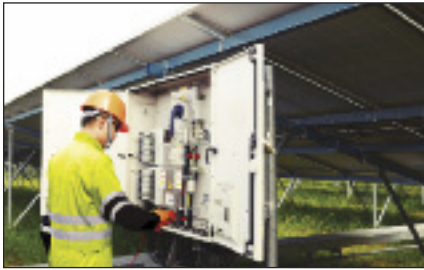
Extreme X provides a high arc-protection rating for workers in such as power stations.
